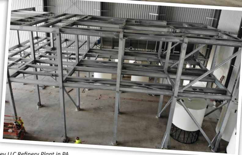
OMNIS Bailey LLC Refinery Plant in PA
