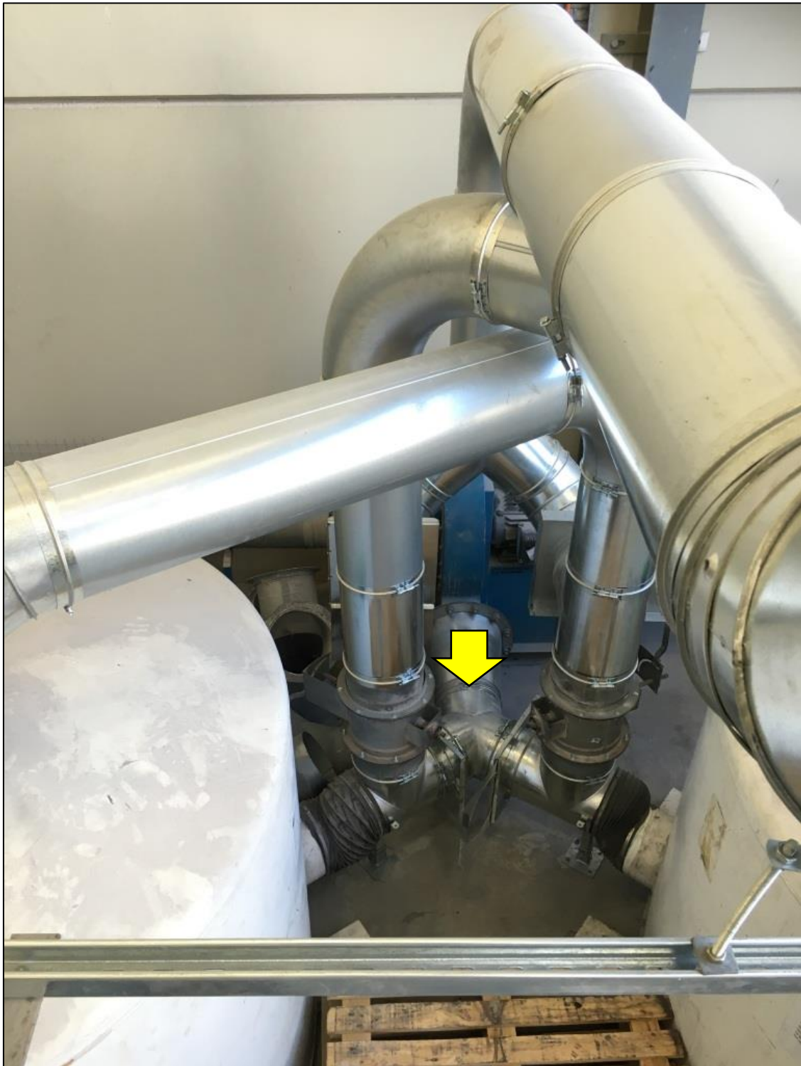
PHOTOGRAPH 2 VARIABLE SPEED FAN EXTRACTING AIR FROM WITHIN PLANT TO SCRUBBER TOWERS IN SERIES
