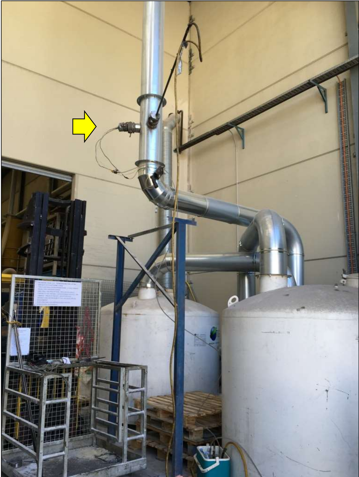
PHOTOGRAPH 1 DRY CARBON SCRUBBERS AND OUTLET SAMPLE PORTS
